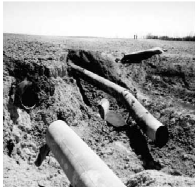
Ruptured Lines 100-3 and 100-4
