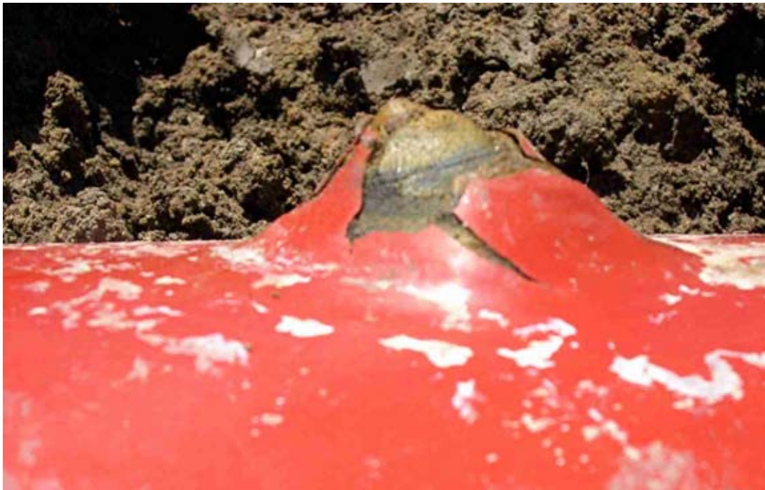
FIGURE 12: Typical AC Assisted Corrosion Product Formation
