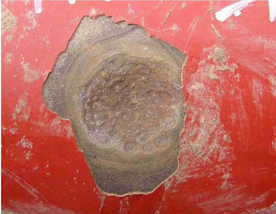
FIGURE 13: Figure 12 with Corrosion Product Removed
