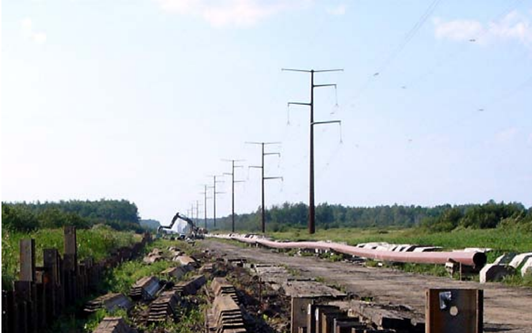
FIGURE 3: Example of HVAC Hazard during Pipeline Construction in HVAC ROW
