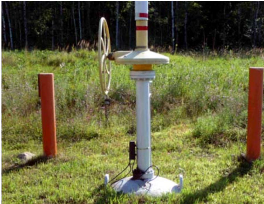
FIGURE 20: DC Decoupler at Mainline Valve Ground Mat
