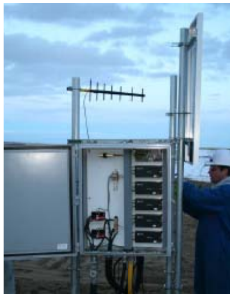
FIGURE 5 - Remote Monitoring Station (RMS) shown with the cabinet door open. Electronics are housed in a NEMA 4X enclosure and are connected to a solar panel and cellular antenna.
