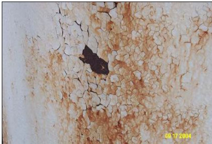
FIGURE 27 – Close view of Figure 26 showing severe coating degradation.
