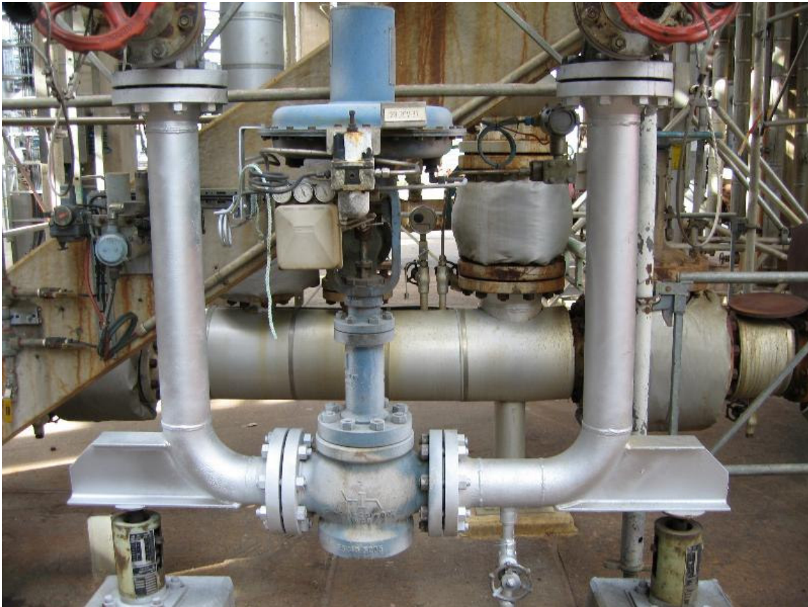
FIGURE 23 – Sweden refinery piping coated with TMIC.
