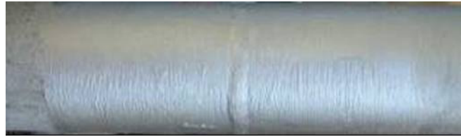
FIGURE 15 – Welded pipe joint after application of TMIC over bare steel and TSA.
