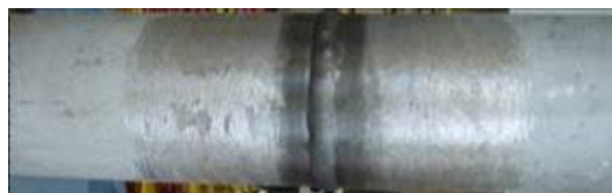
FIGURE 13 – TSA coated pipe with welded joint.
