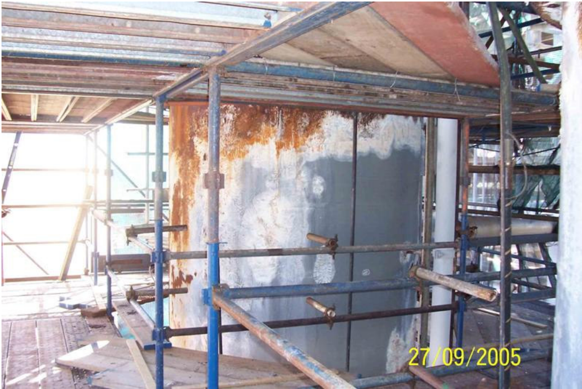
FIGURE 18 – Propane Treater Vessel – Failure of IOZ and subsequent CUI.
