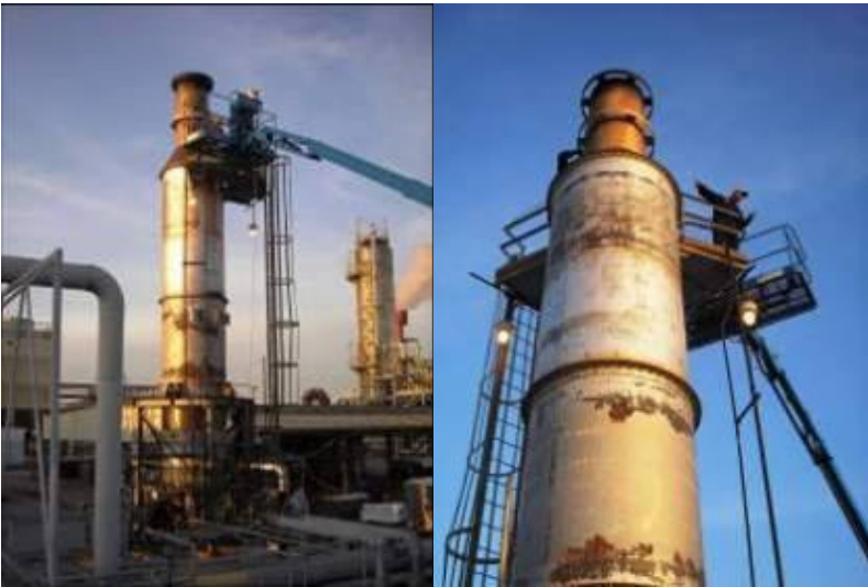
FIGURE 21 – Incinerator after CUI failure
