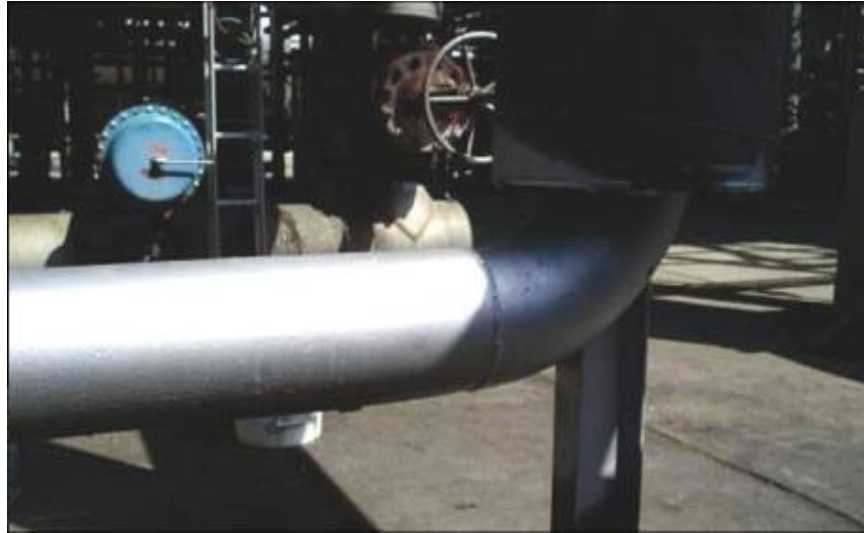
FIGURE 24 – Sweden Refinery Piping – condition of TMIC after 2.5 years service.
