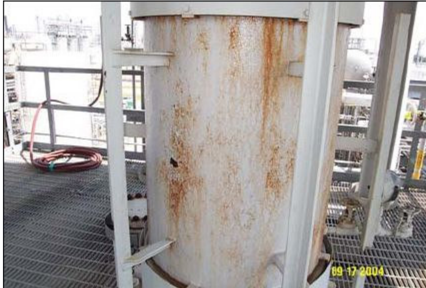
FIGURE 26 – Texas refinery gas dryer unit showing breakdown of traditional high heat coating after 12 months in service.
