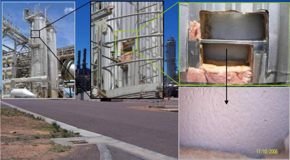
FIGURE 20 – Propane Treater Vessel –inspection of TMIC condition after 1 year service.
