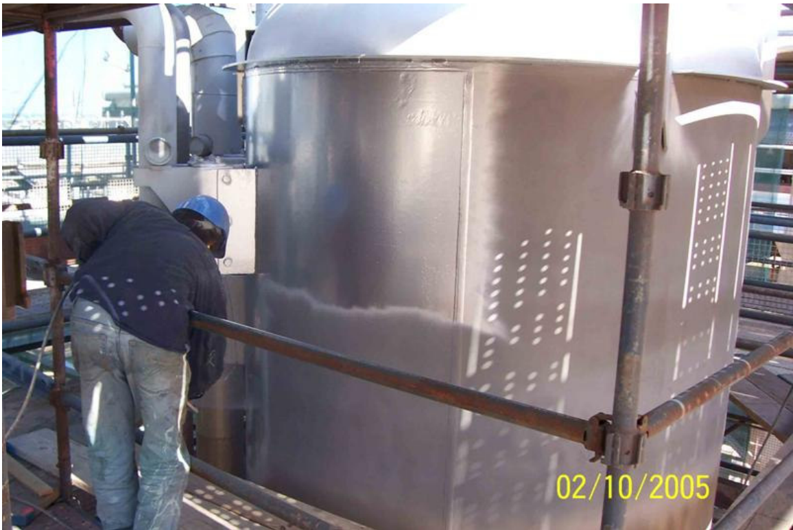
FIGURE 19 – Propane Treater Vessel – TMIC being applied.
