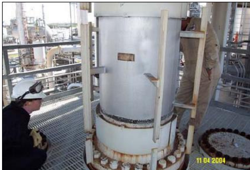
FIGURE 29 – Inspection of TMIC after 1 year in service showing no coating breakdown or rusting.
