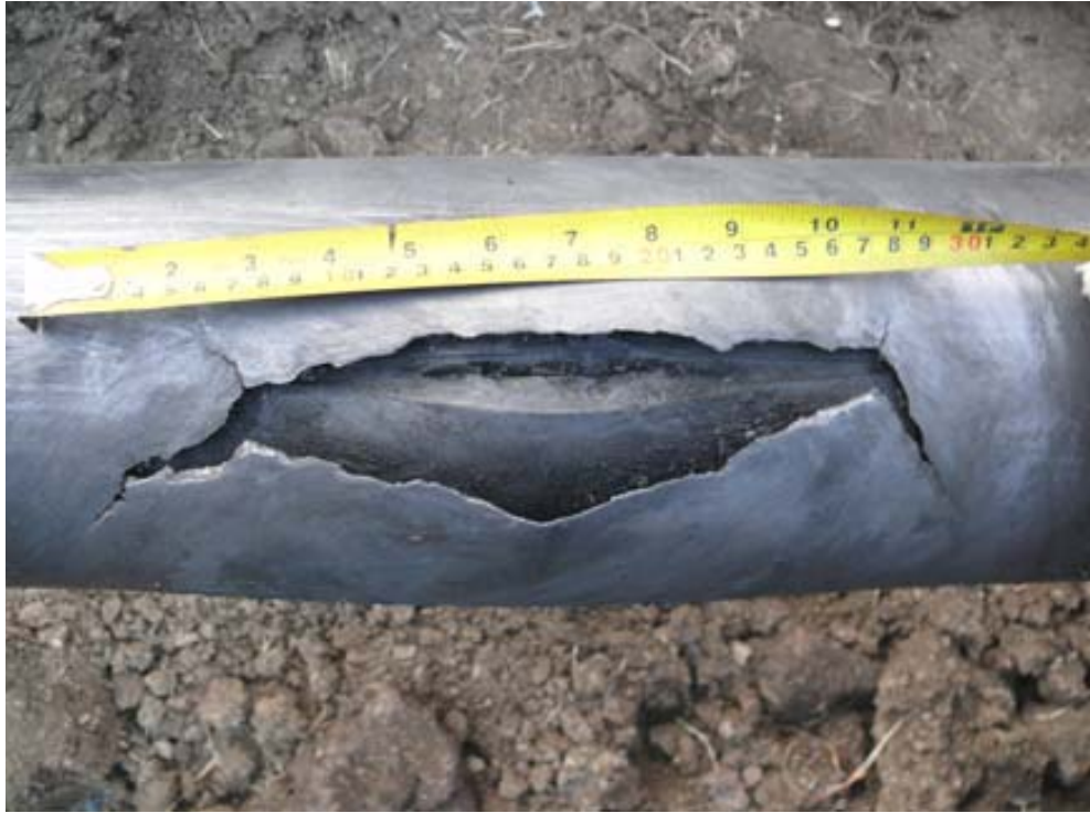
FIGURE 1 - Failure after insulation and coating removal
