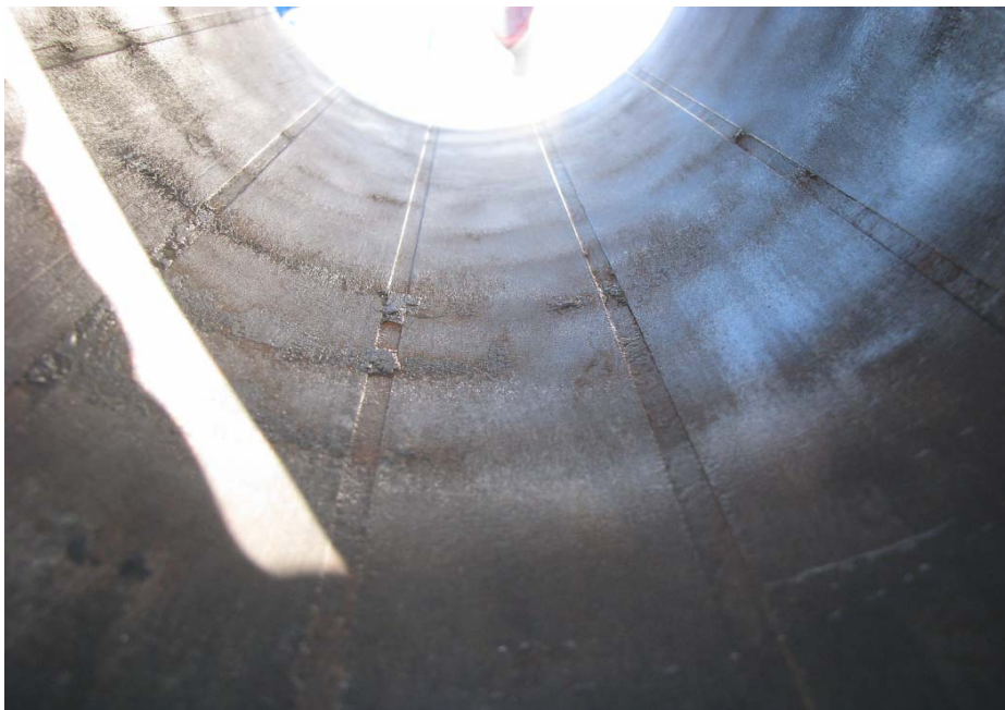
FIGURE 6 - Shallow Corrosion on Steel Pipe ID Adjacent to External Grooves in HDPE Liner
