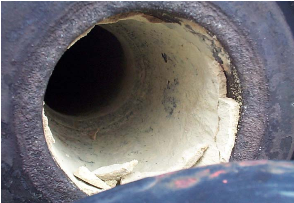
S 8 deposition within a sour gas flow line +
