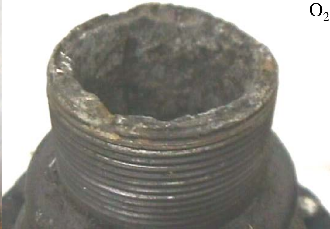
Corroded Stuffing Box
